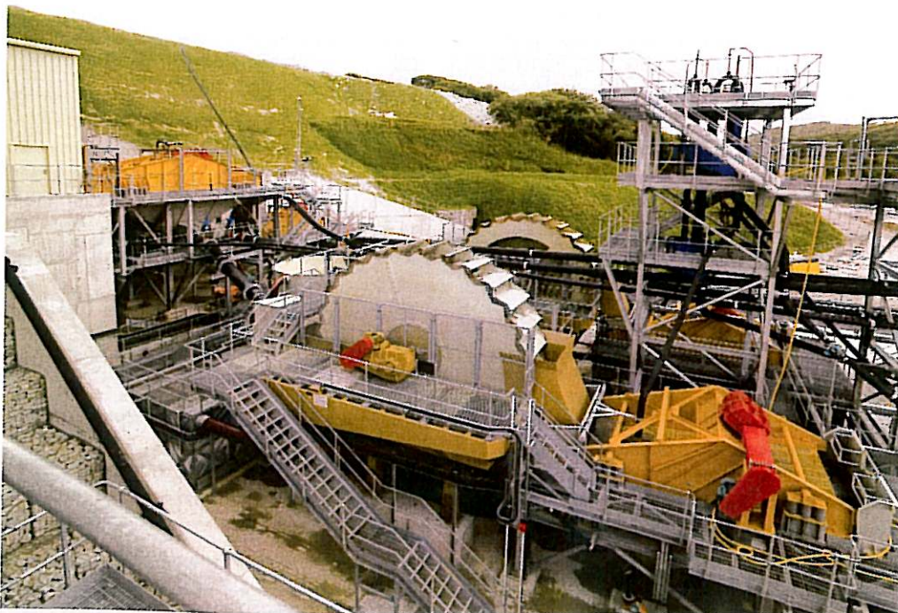
The sand-separation system comprises two bucket wheels and two dewatering screens
